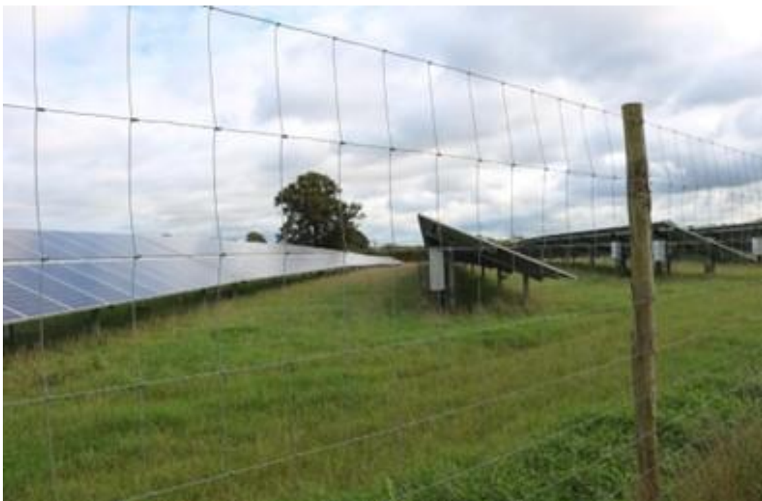
Deer-proof post-and-wire fencing at solar site in Worcestershire
